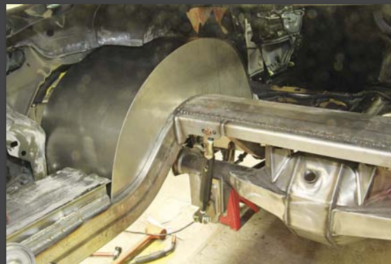
■ David and Greg Engle fabricated the massive inner wheel-well tubs and rear back-half frame clip and trunk floor sheet metal.
